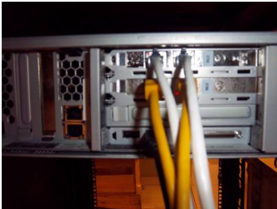
Figure 11: GigE Connections from Distance Emulator to Brocade Fabric
